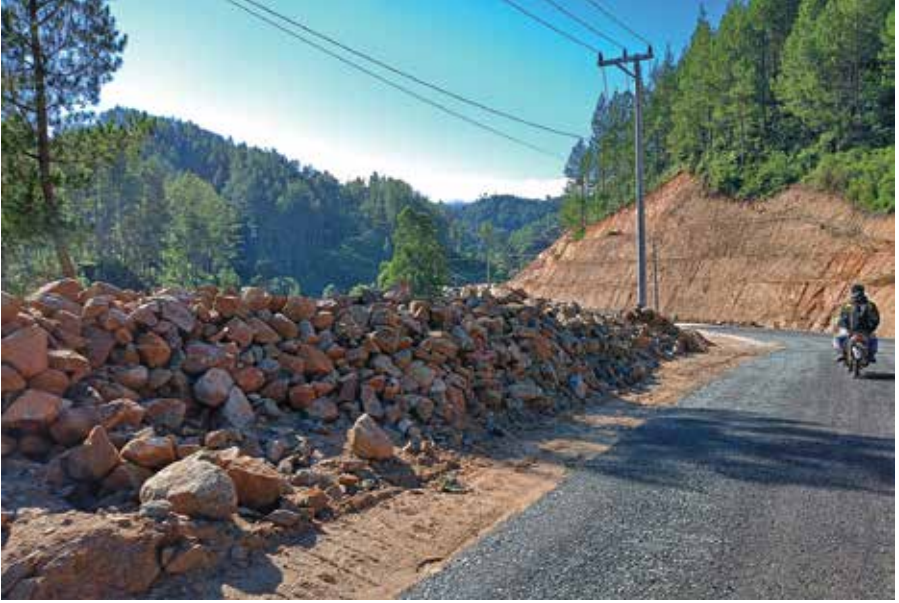
Figure 43 An ongoing road expansion will threaten at least three species of Rhododendron , i.e. R. celebicum , R. tjiasmantoi , and R. zollingeri . The construction is still in the lower part of Pasapa' Lombonan and is expected to be finished before mid-2024.
